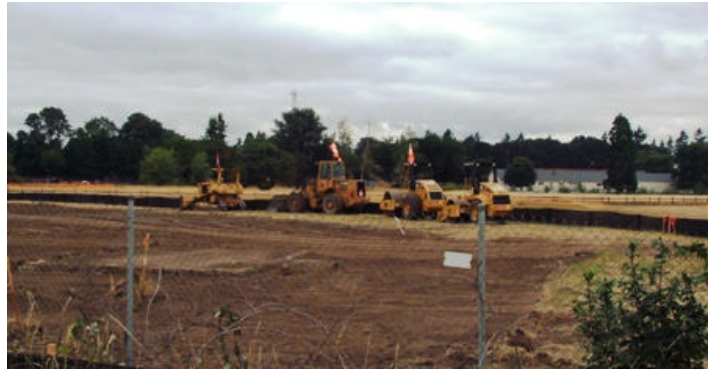
Kiewit Pacific machinery lines up along Highway 14 where crews are preparing for construction of Maya Lin bridge connecting historic reserve with Columbia River waterfront. Expected completion date is August 2007.
